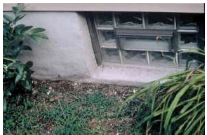
FIGURE 15.2 Visible paint chips and debris in the soil.
