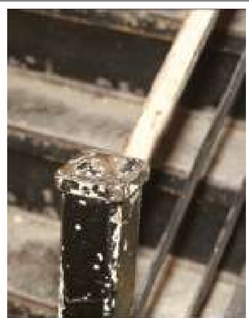
FIGURE 12.5 A metal railing before abatement.
