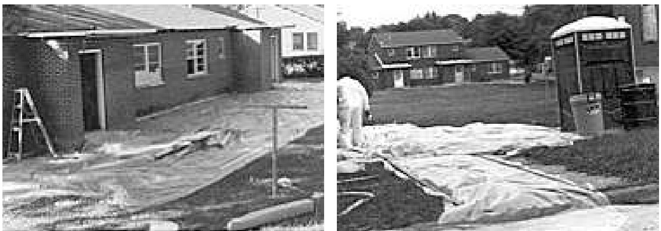
FIGURE 12.8 Line surfaces with plastic in the work area (left) and pathways (right)
