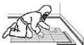
FIGURE 12.10 Install underlayment and new flooring as a suitable LBP enclosure method. The personal protective equipment is for a high-dust project.
