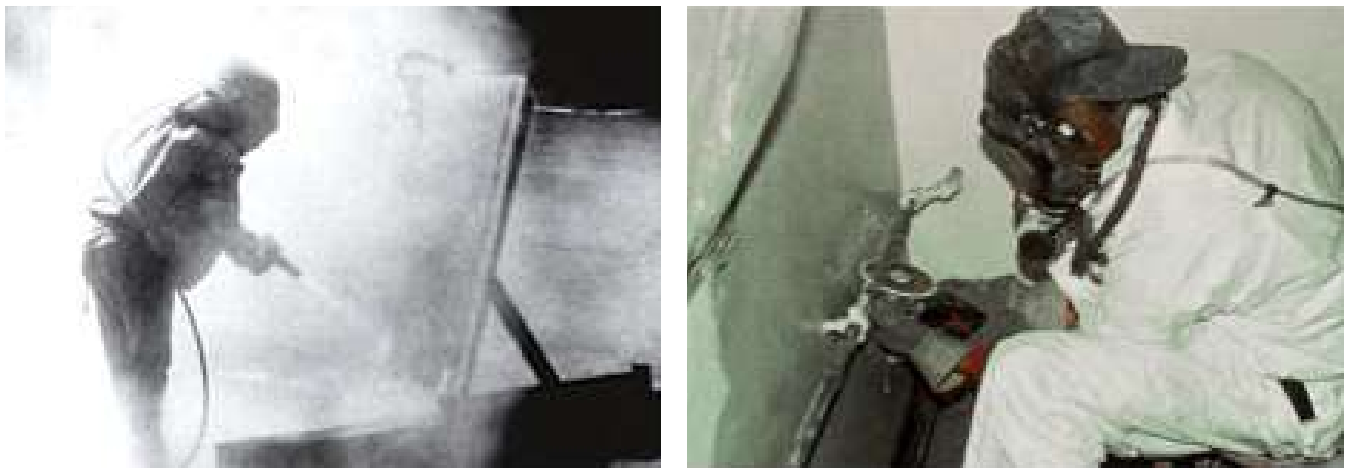
FIGURE 12.13 Prohibited work practices (traditional abrasive blasting (left) and grinding without HEPA exhaust).
