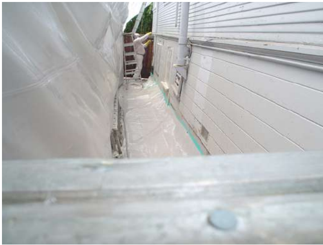
FIGURE 8.14 Exterior containment of polyethylene sheeting lines the narrow walkway between two houses. Notice the abatement worker in the background.
