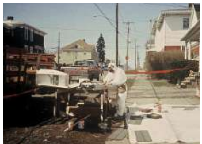
FIGURE 12.7 Certified workers are needed to replace siding when the project's intent is lead abatement.
