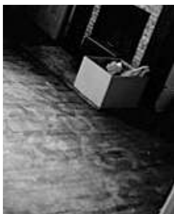
FIGURE 15.3 Visible Dust Indicates Recleaning is Needed
