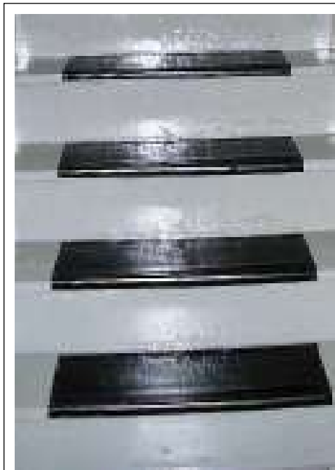
FIGURE 5.6b Friction hazard on stairs post-treatment.
