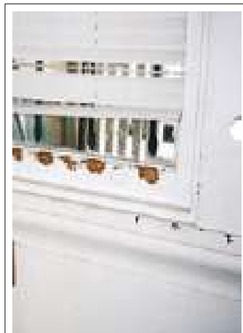
FIGURE 5.8 Chewable surface: teeth marks on window sill.
