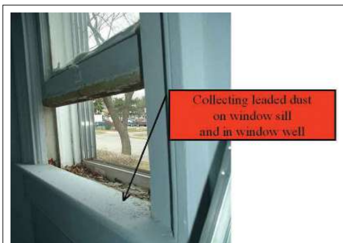
FIGURE 5.13 Window sill (at arrow); trough is behind sill, under sash and in front of storm window tracks.
