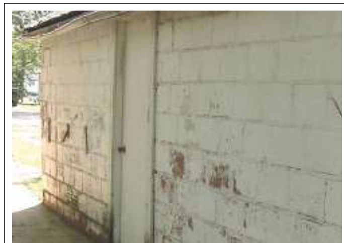
FIGURE 5.10 Soil lead hazard at dripline of garage.
