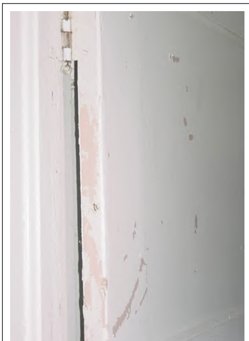
FIGURE 5.7 Impact surface on door and frame.
