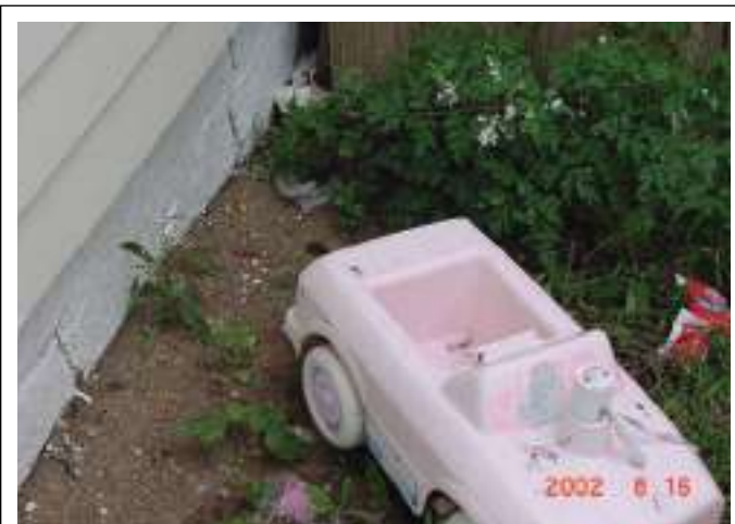
FIGURE 5.9 Soil lead hazard at dripline
