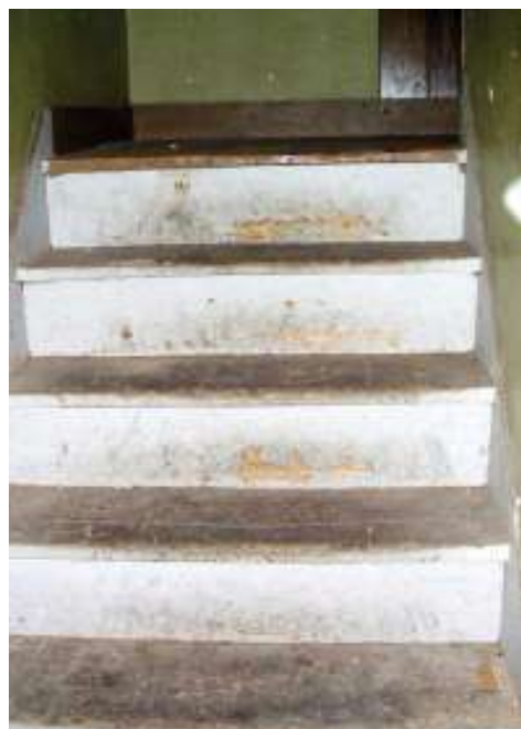
FIGURE 5.6a Friction hazard on stairs pre-treatment.
