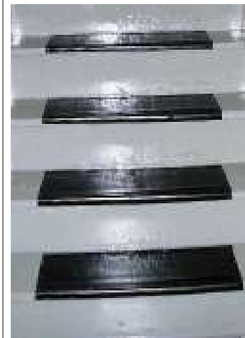
FIGURE 5.6b Friction hazard on stairs post-treatment.
