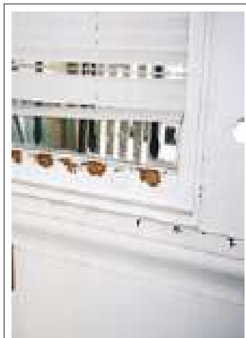
FIGURE 5.8 Chewable surface: teeth marks on window sill.
