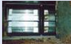
Photo 4C: Moldy air duct
