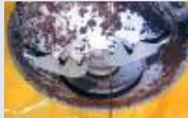
Photo 4B: Mold growth on air diffuser in ceiling
