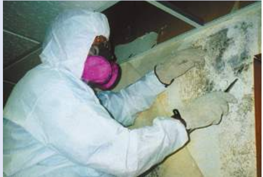
Photo 7: Remediation worker with limited PPE
