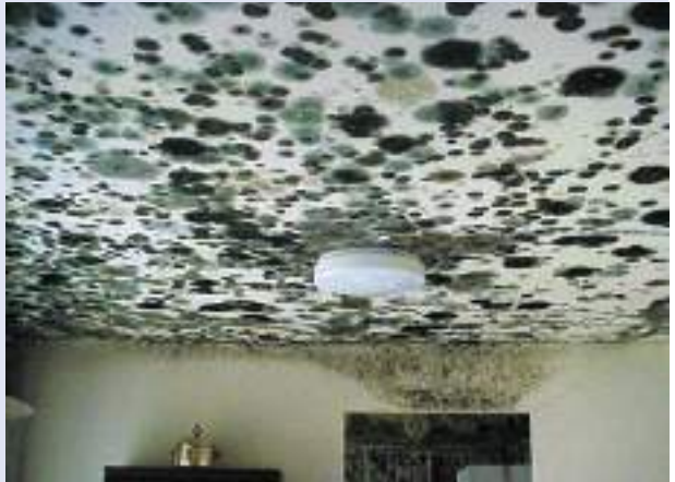
Photo 2: Extensive mold contamination of ceiling and walls
