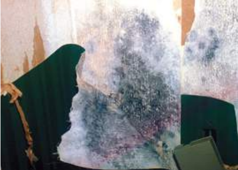
Photo 5: Mold growth behind wallpaper
