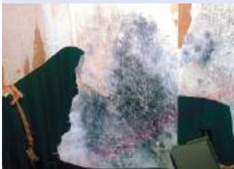
Photo 5: Mold growth behind wallpaper
