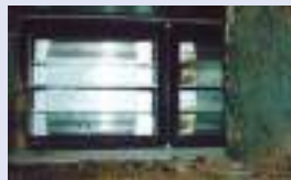
Photo 4C: Moldy air duct
