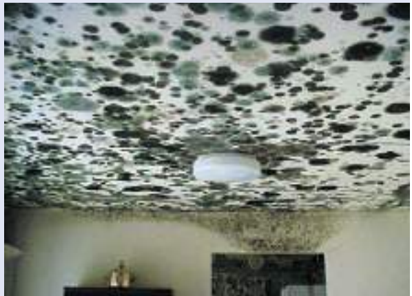
Photo 2: Extensive mold contamination of ceiling and walls
