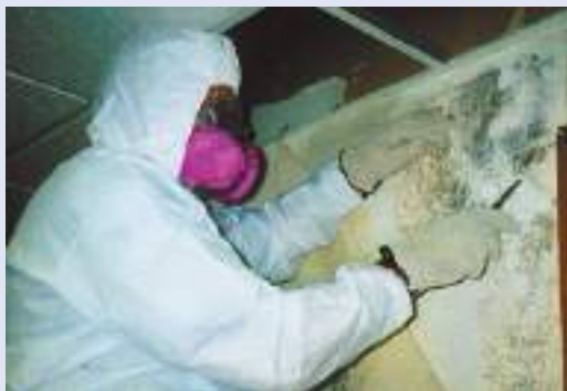
Photo 7: Remediation worker with limited PPE
