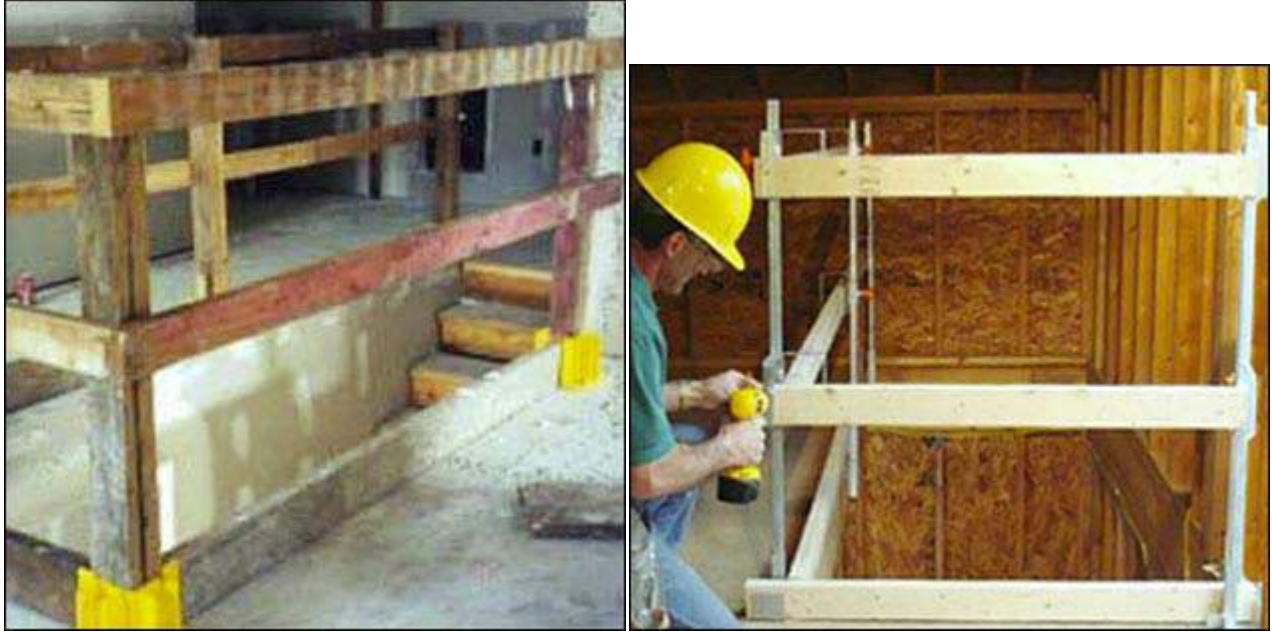
Figures 21 & 22 - Examples of guardrails installed around floor openings.
