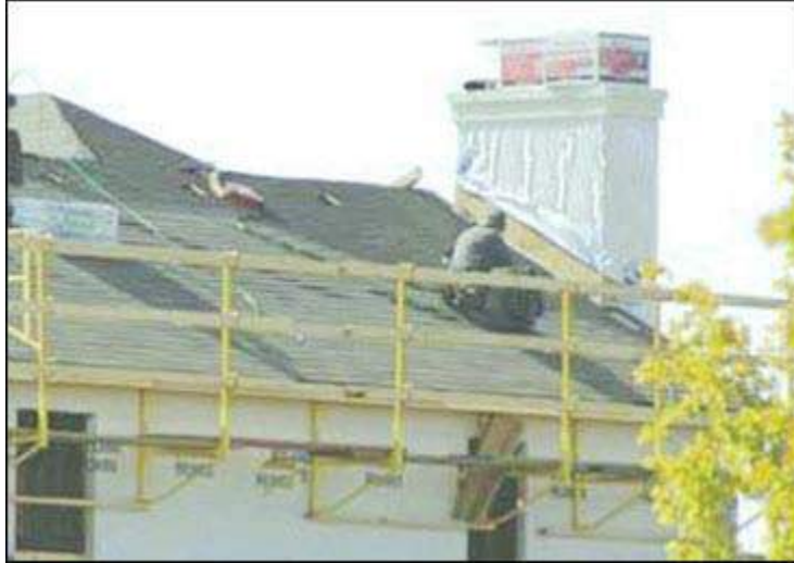
Figure 10 - An exterior bracket scaffold with guardrails being used to protect workers while weatherproofing.
