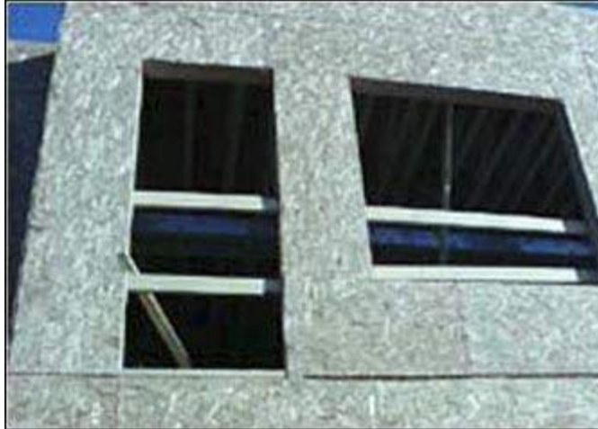
Figure 35 - Guardrails protecting window openings.
