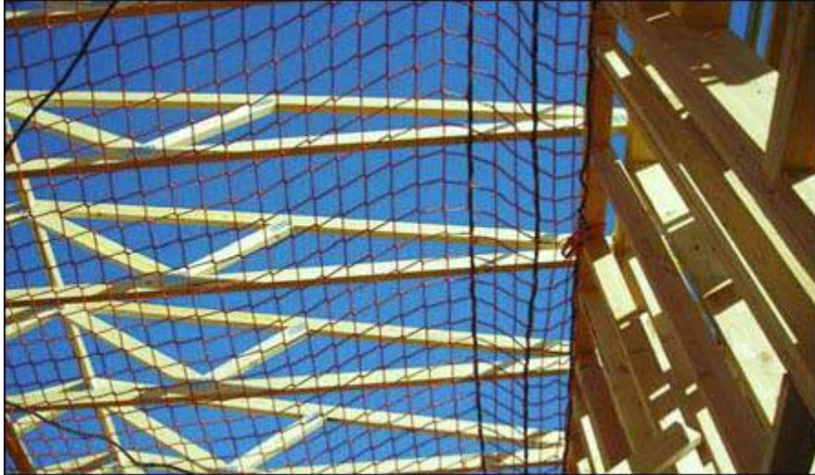
Figure 7 - An example of a safety net system.
